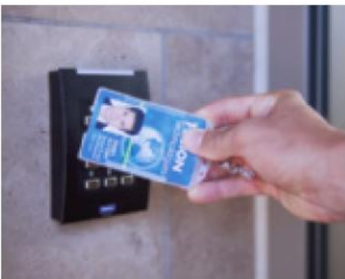
ACCESSING A SECURE FACILITY VIA A CONTACTLESS SMART CARD READER
